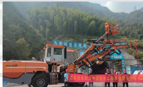
UJ22 浙江·蓄能电站 UJ22 Zhejiang · Pumped hydropower station
